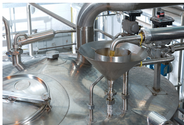
Fig. 2 Typical Food Production Equipment
